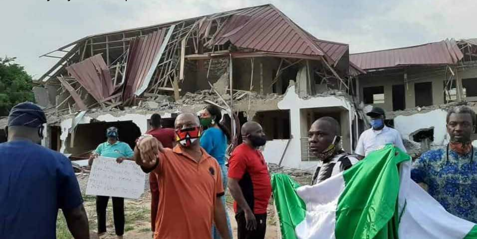
The Nigerian High Commissioner's residence in Accra that was unlawfully razed down
